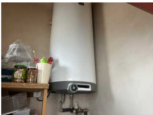
el. boiler ve spíži
